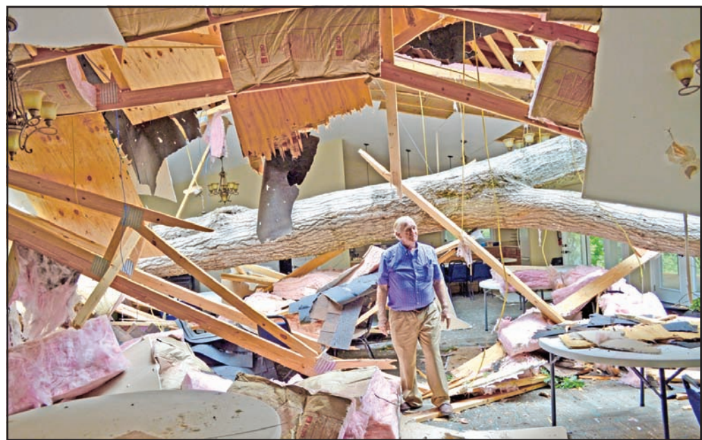
Morris Phillips standing inside the fellowship hall of Friendship Baptist Church in Hiawassee, after a big tree wrecked the building on Sunday, June 24. Photo by Lowell Nicholson
